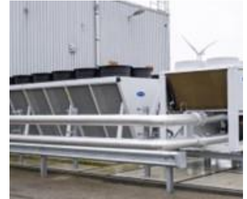
Heat pumps in Cell Culture Media Factory
