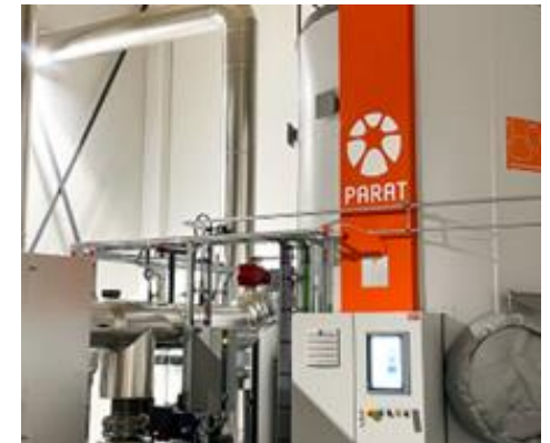
Installation of E-boiler
