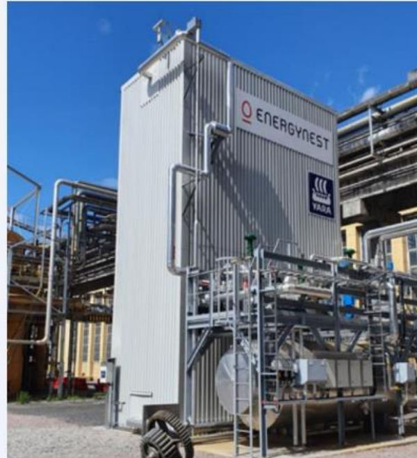
EnergyNest - Yara (No) TES for steam grid balancing
